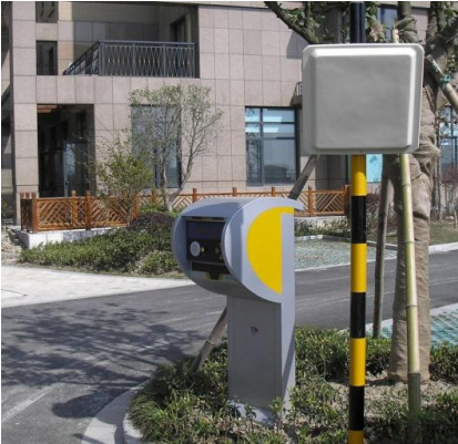
Pole Mounted Antenna
